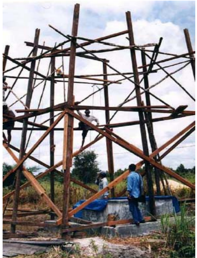
Construction of one of the two towers built by IRDN in cooperation with Rungan Sari engineers
